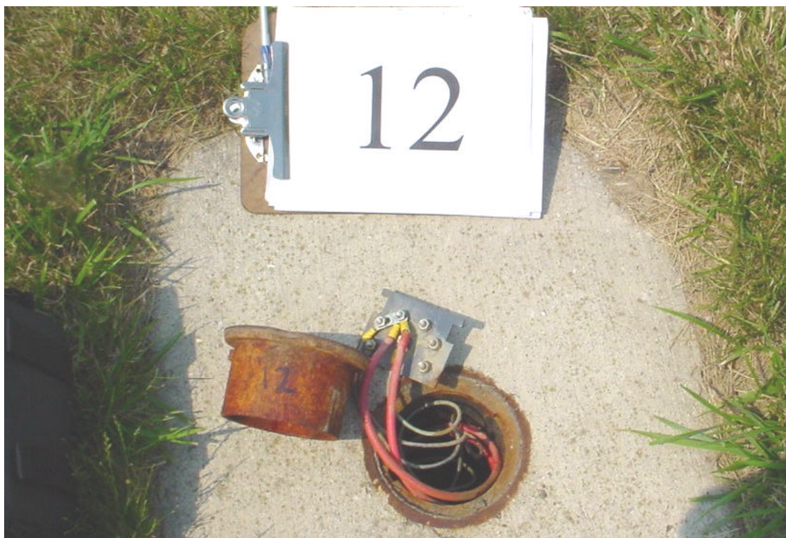
Figure 31 - Test Station #12, close-up
