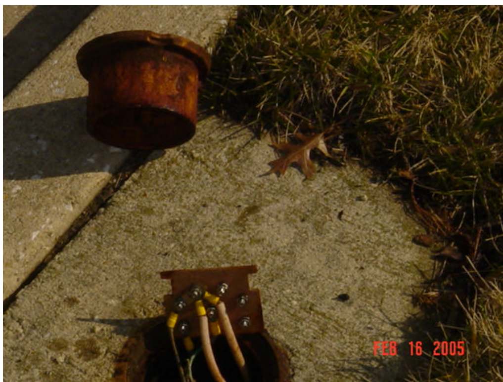
Figure 150 – Test Station 12 close up
