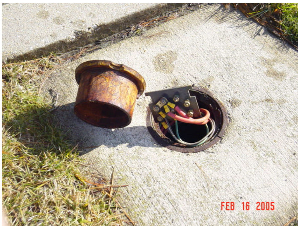
Figure 142 – Test Station 8 close up
