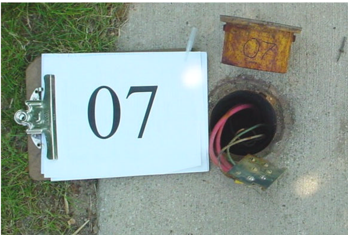
Figure 21 - Test Station #7, close-up
