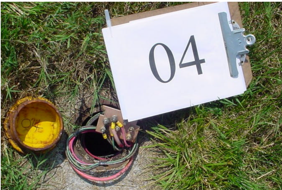
Figure 15 - Test Station #4, close-up
