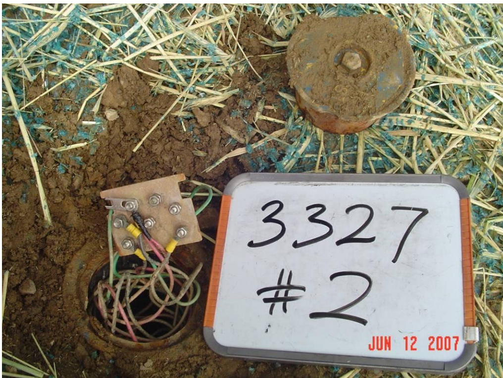
Figure 124 - Test Station 2 close-up
