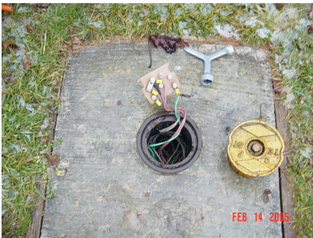
Figure 130 - Test Station 2 close-up
