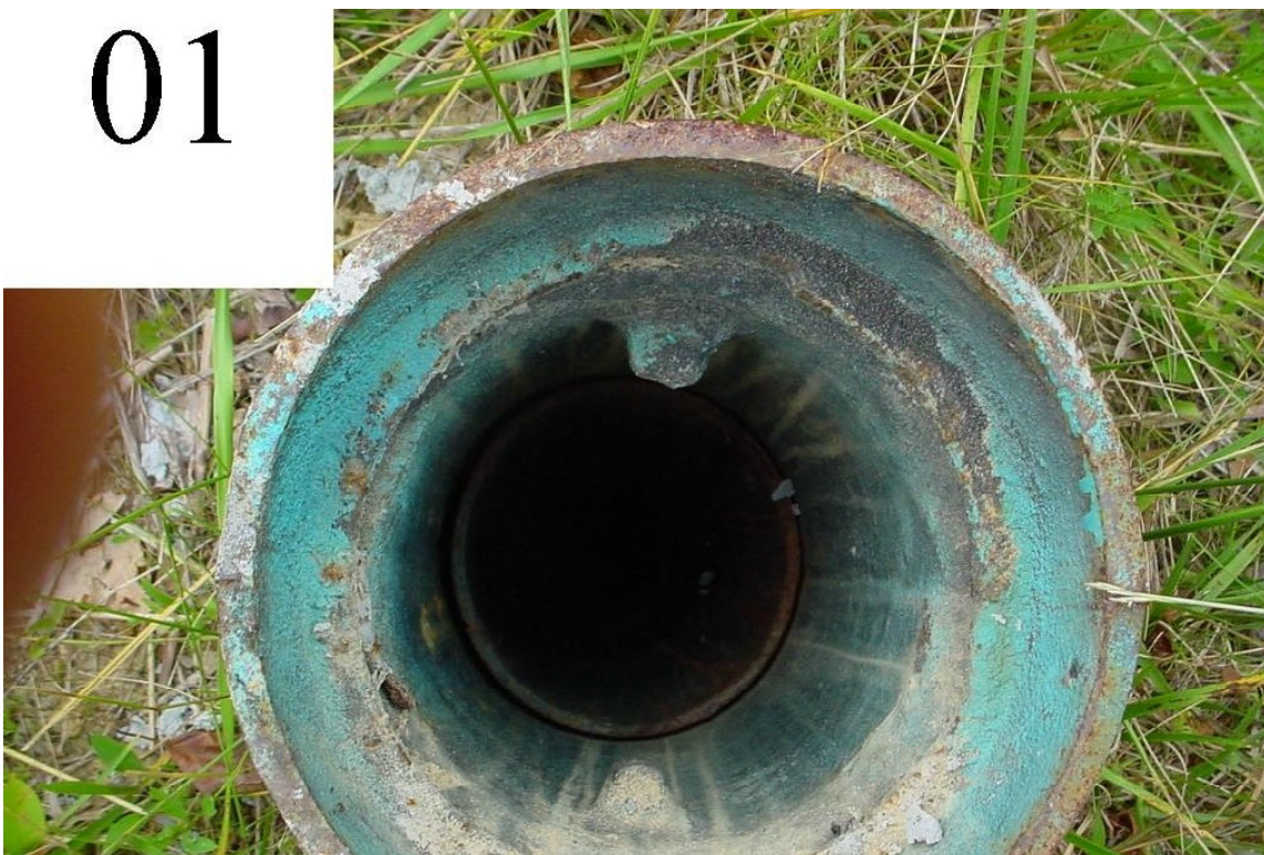
Figure 9 - Test Station #1, close-up
