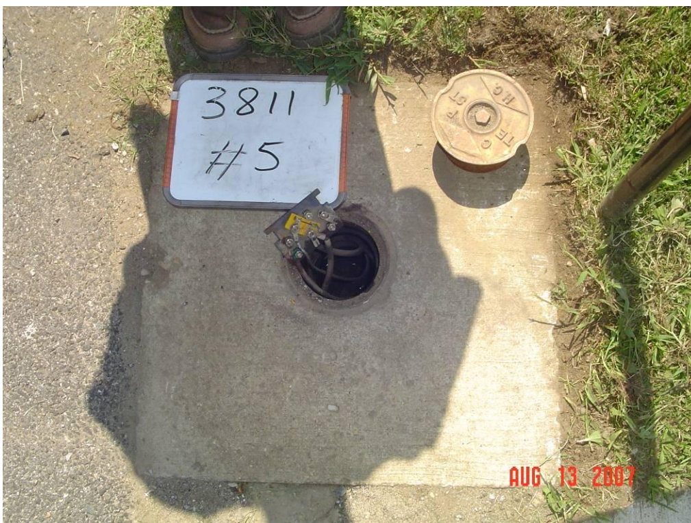
Figure 193 - Test Station 3811-5 close-up
