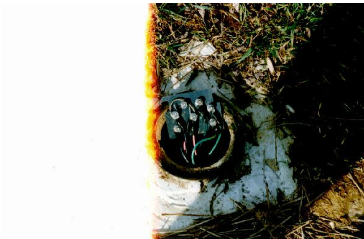
Figure D - 8. Close-up of Test Station No. 04
