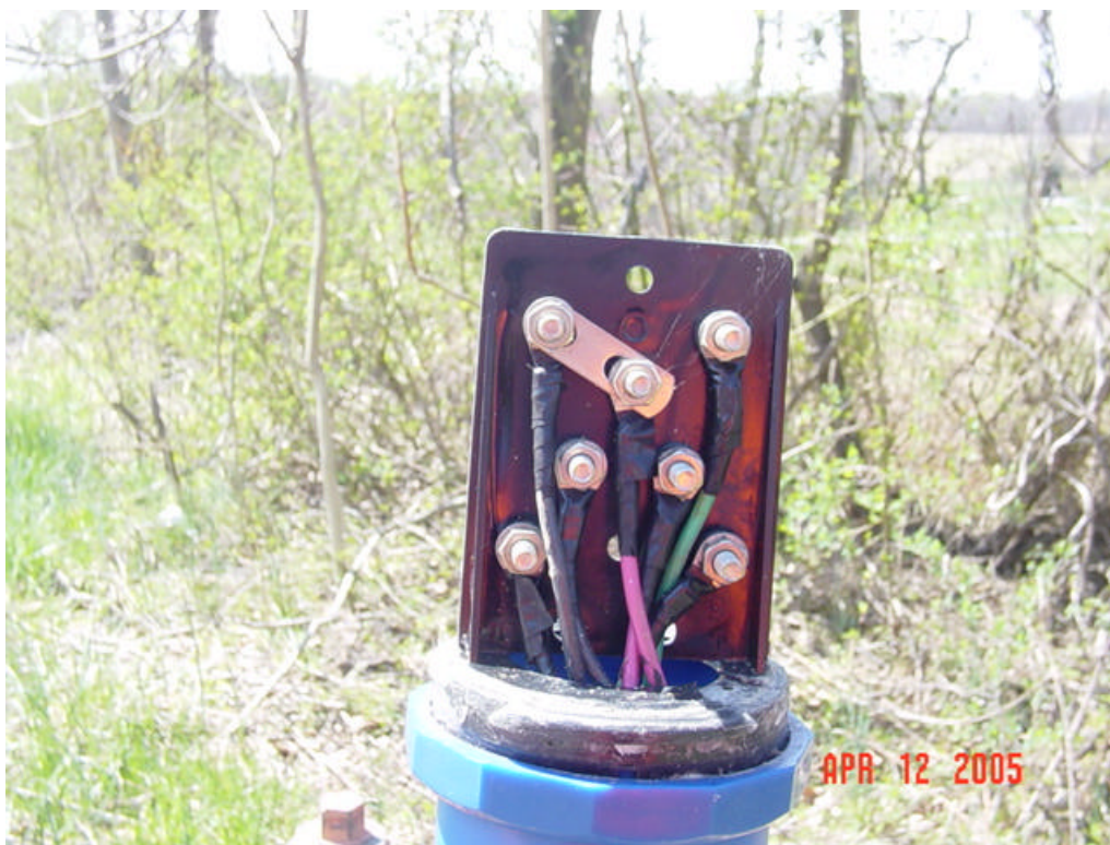
Figure 231 - Test Station 3480-4 close-up
