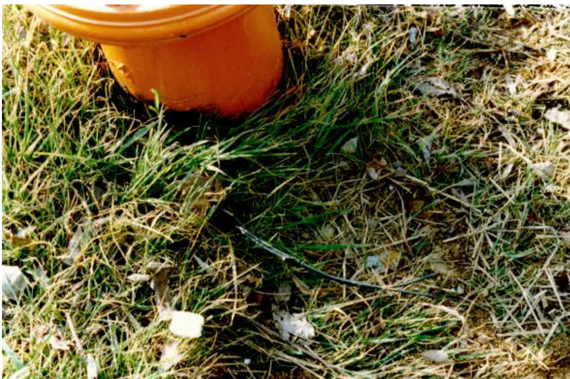
Figure D - 4. Close-up of Test Station No. 02
