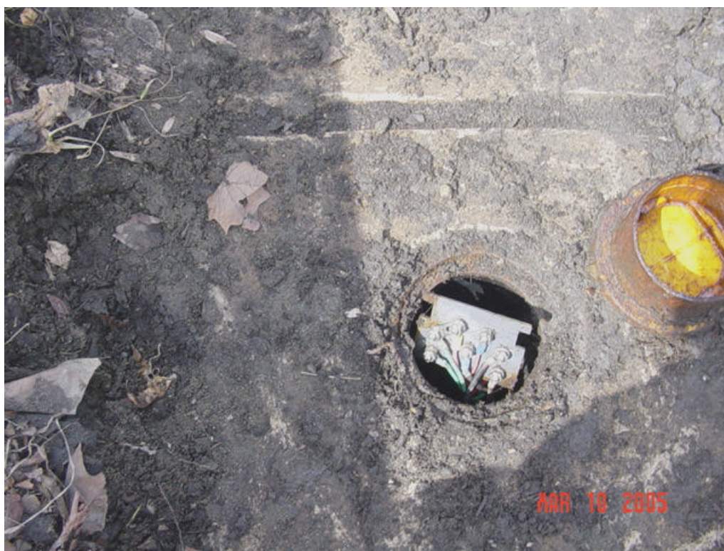
Figure 72 - Test Station 8W-1 close-up
