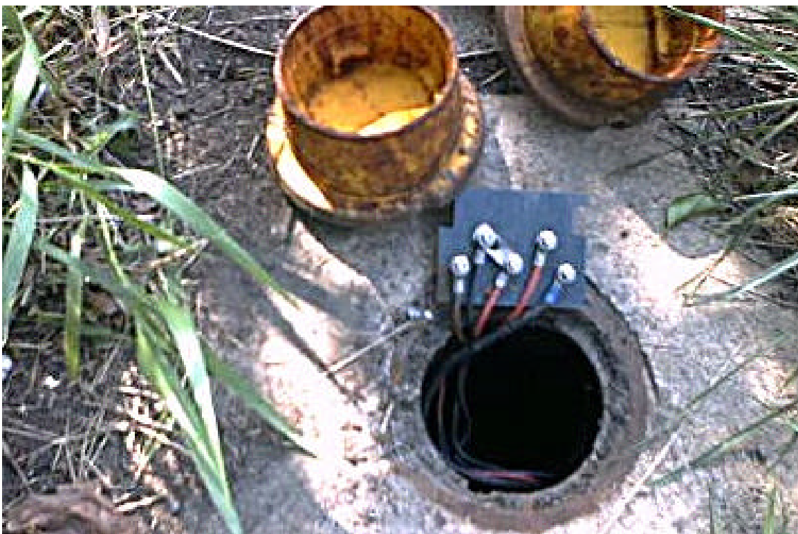
Figure 79 - Test station #1, close-up
