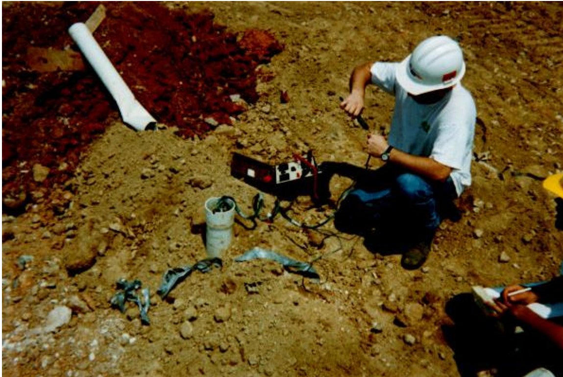
Photo 15. Test Station North of MD108 Overpass
