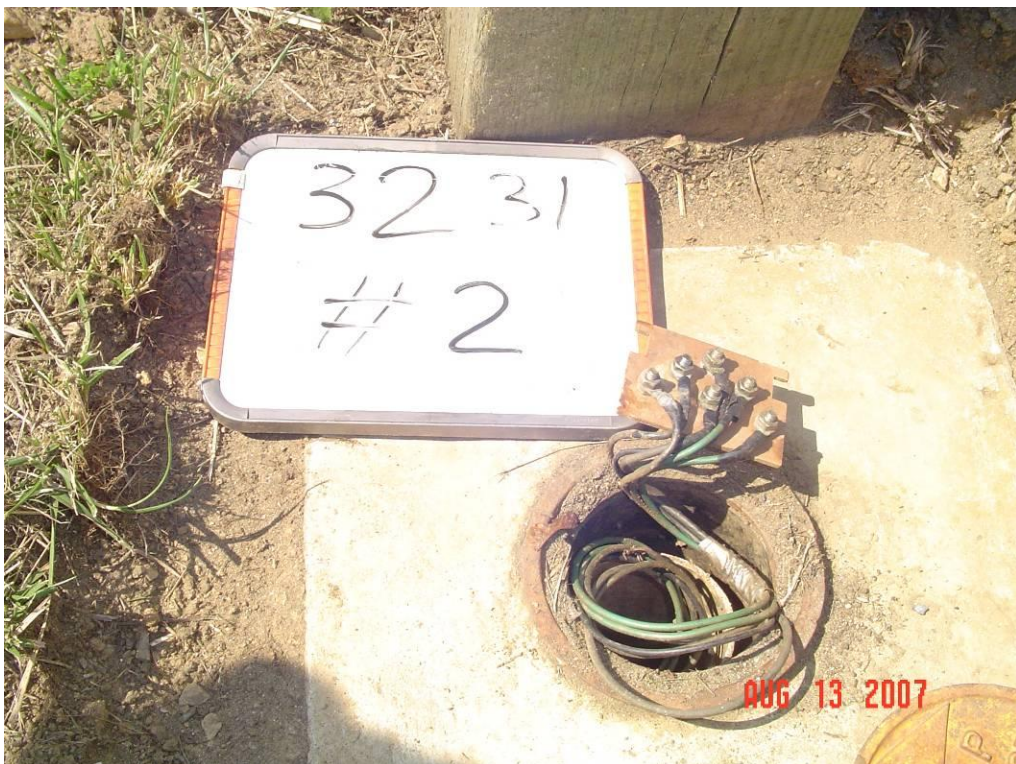
Figure 106 - Test Station 3231-2 close-up
