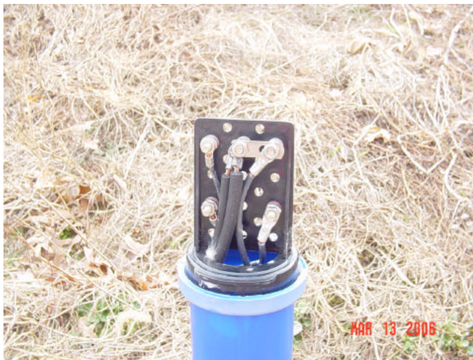
Figure 4 – Test Station 1 close-up
