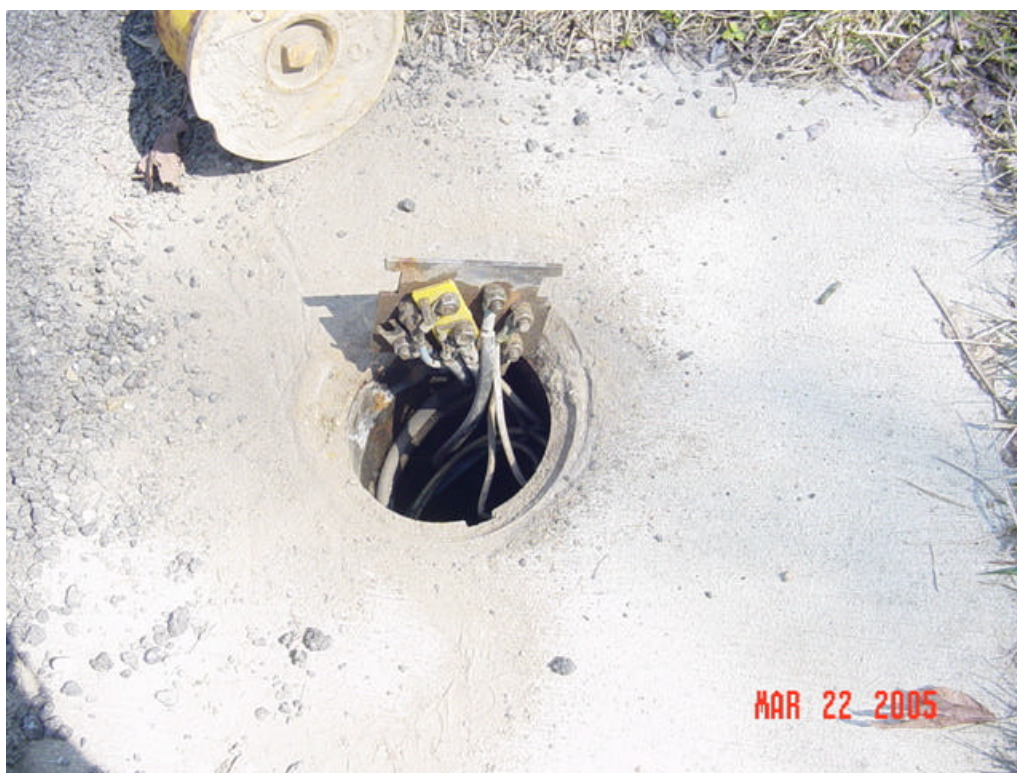
Figure 200 - Test Station 3811-2 close-up
