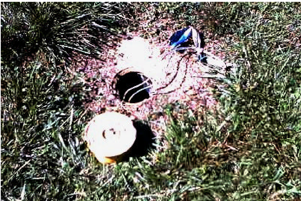
Figure 41 - Test station 8WM2, close-up
