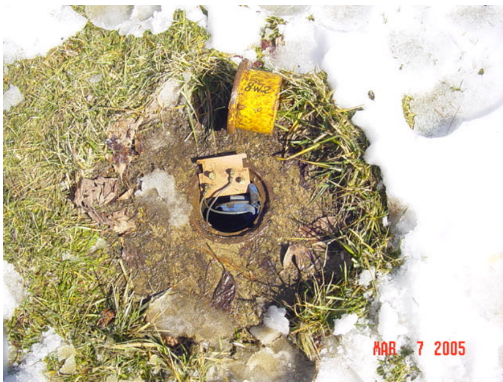
Figure 8 - Test Station 8WM2 close-up
