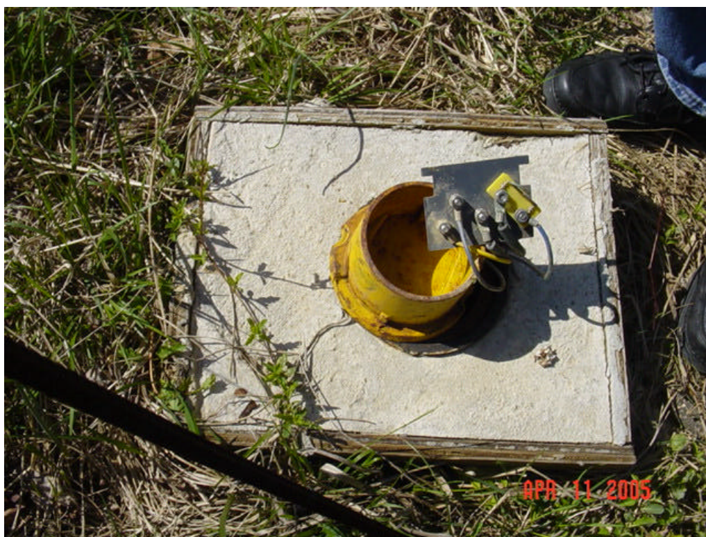
Figure 62 - Test Station 4153-2 close-up
