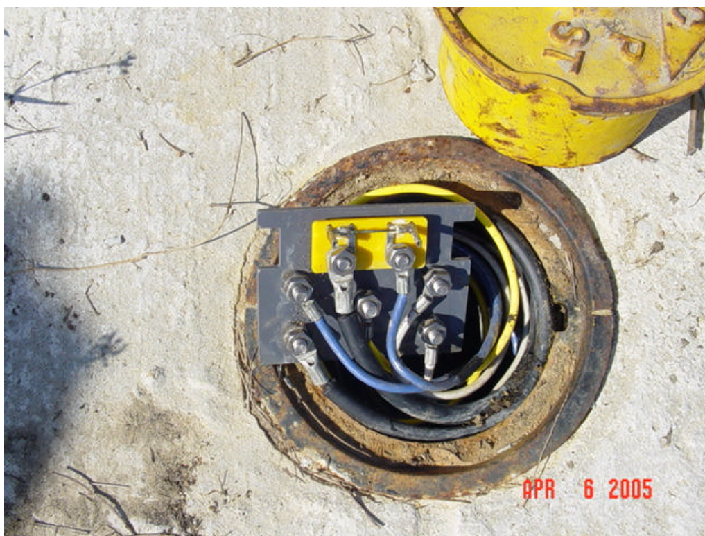
Figure 60 - Test Station 4153-1 close-up
