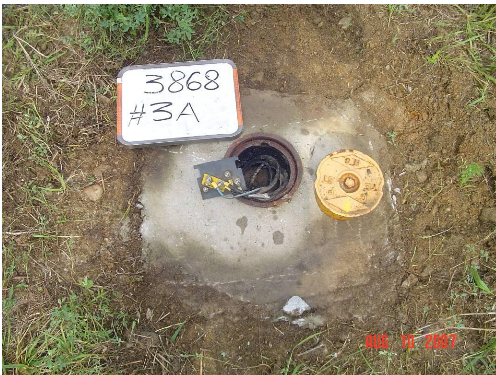
Figure 77 – Test Station 3A close up
