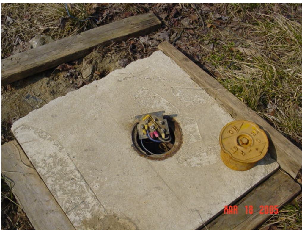
Figure 89 – Test Station 2 close up
