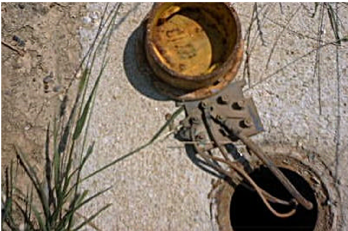
Figure 66 - Test station 175D, close-up
