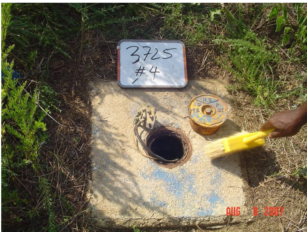
Figure 44 - Test Station 3725-4 close-up
