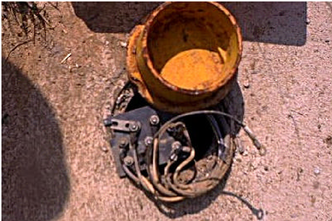
Figure 64 - Test station 175C, close-up
