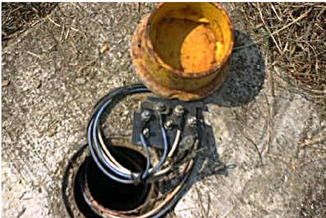
Figure 62 - Test station 175B, close-up
