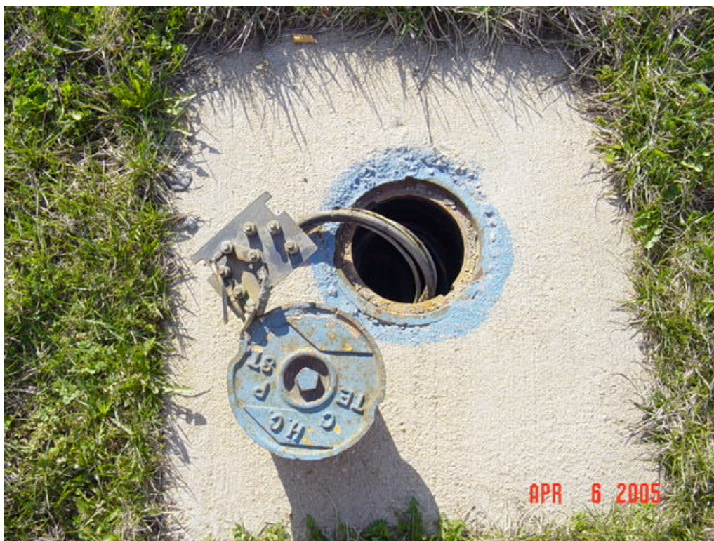
Figure 46 - Test Station 3725-1 close-up
