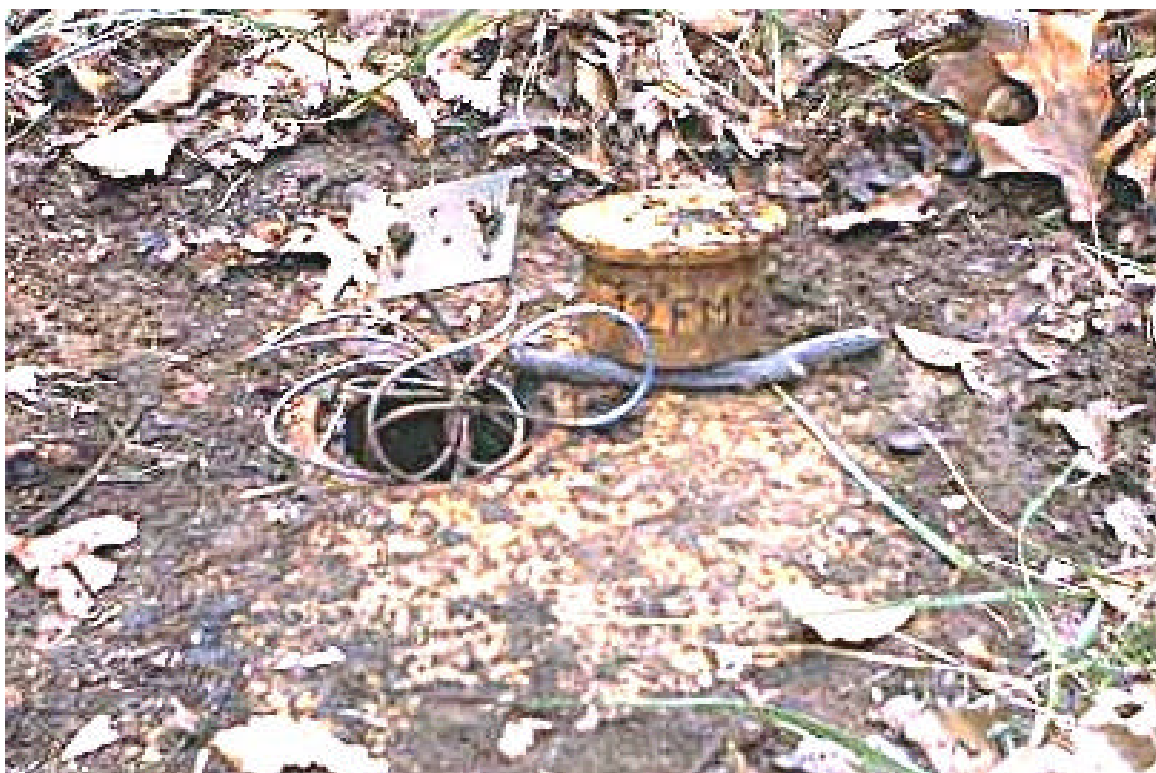
Figure 27 - Test station 12FM8, close-up
