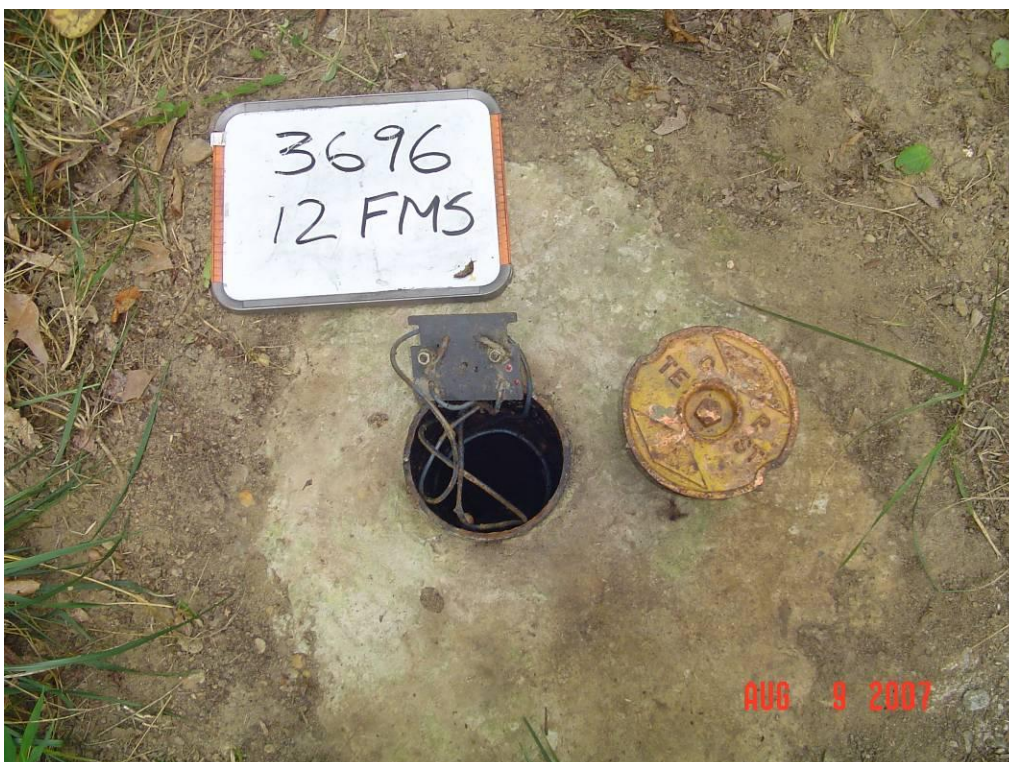
Figure 25 - Test Station 12FM5 close-up
