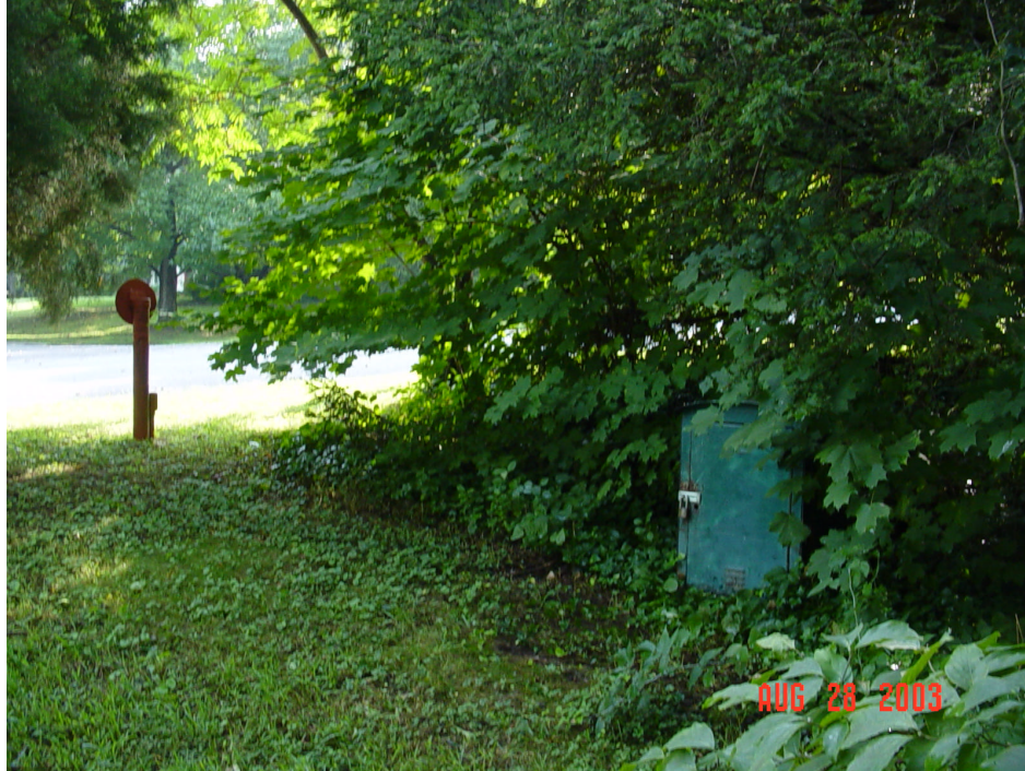
D 6 – Rectifier located on River Meadows Road (N39E20.513', W76E85.420')
