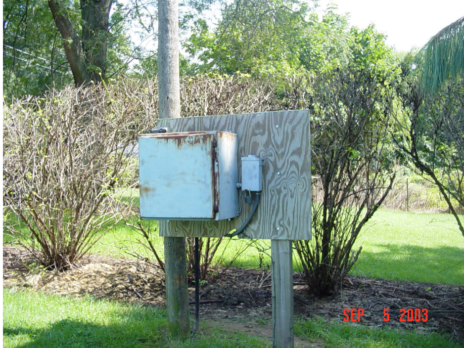
D 5 – Rectifier located near Route 29 and Route 108 (N39E24.099', W76E83.244')
