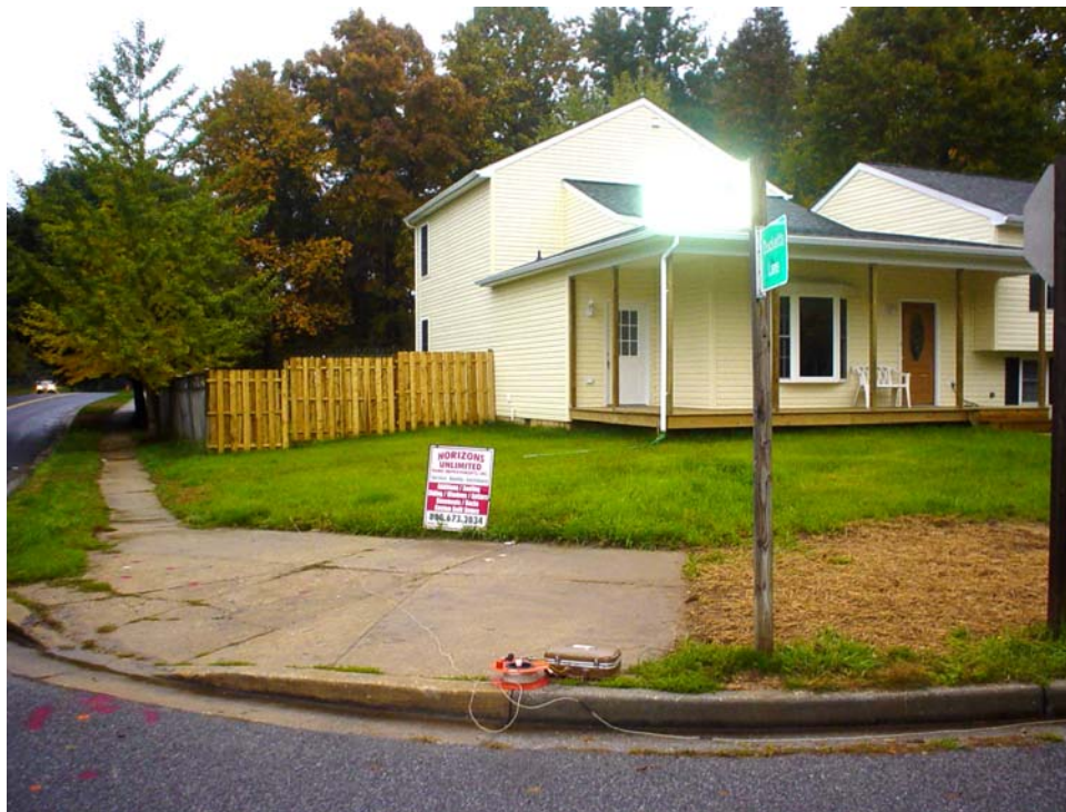
Figure 34 - Stray Current Testing on Ducketts Lane and Kyle Leaf Court
