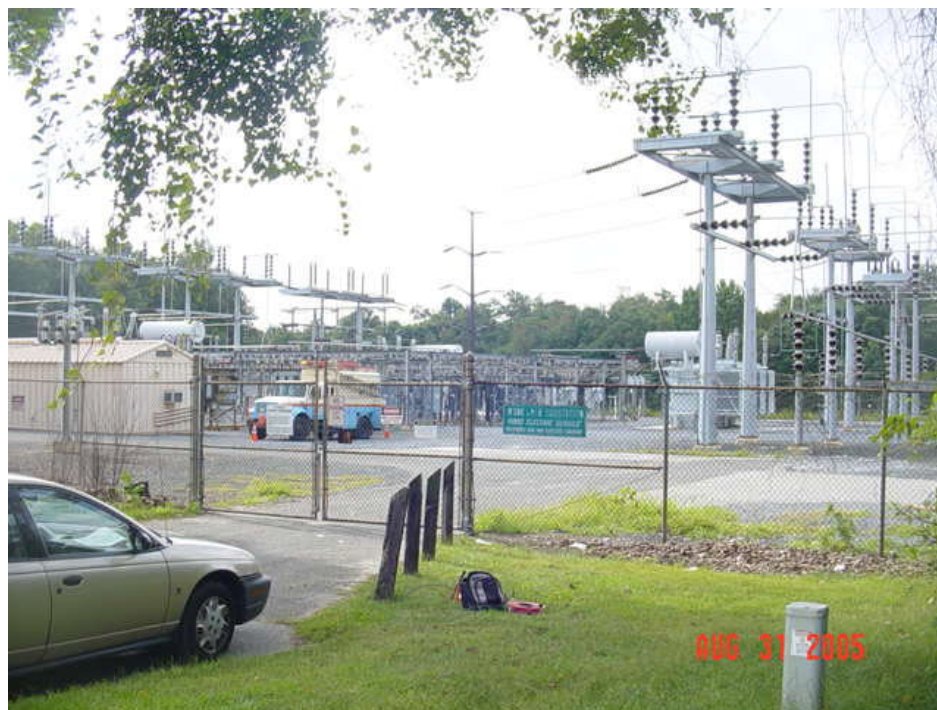
Figure 113 – Wilde Lake substation
