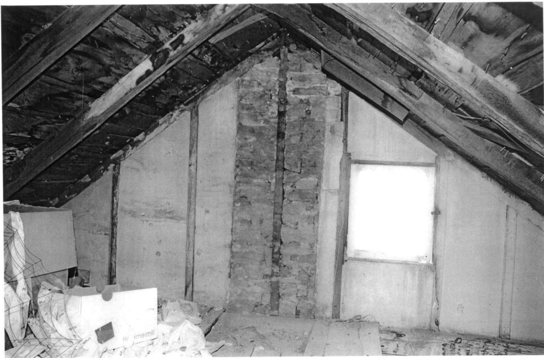
HO-916 "Mount View" Farm 12985 Frederick Road Ell attic, southwest elevation Ken Short, October 2006 7/7
