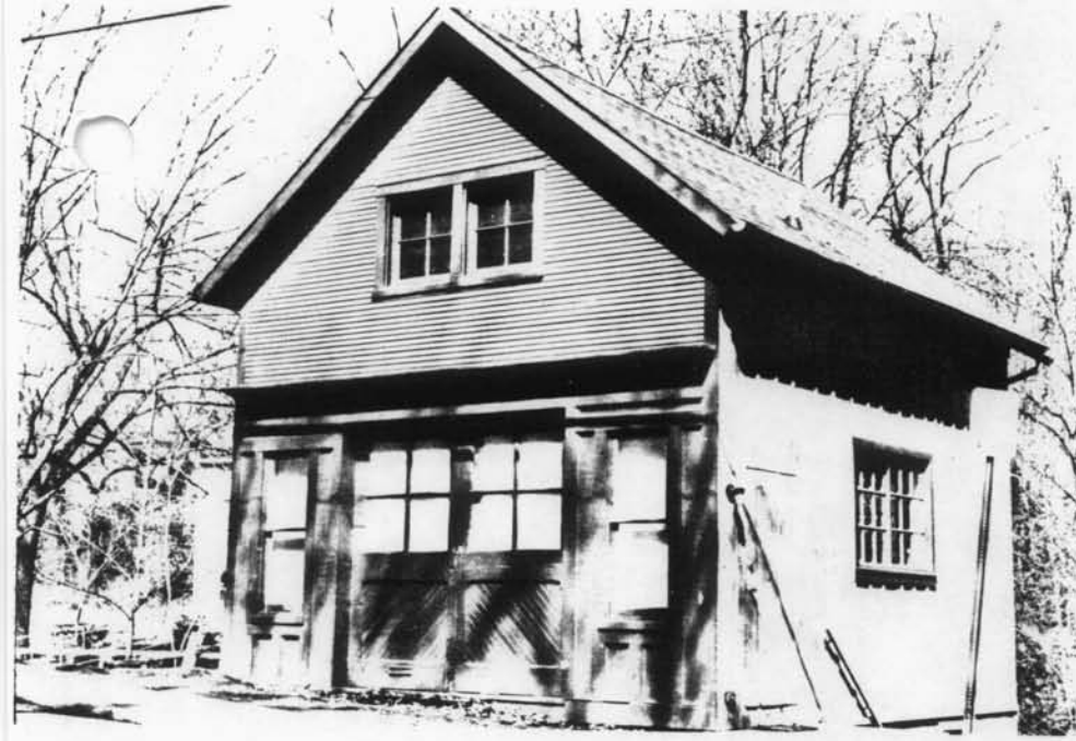
Fig. C-1 Front facade restored using all existing material. Windows and carriage doors repaired. Right side elevation shows new sliding wooden sash with true divided lights to match original plus new "concealed" door used as main entrance. All siding existed pre-rehab.
