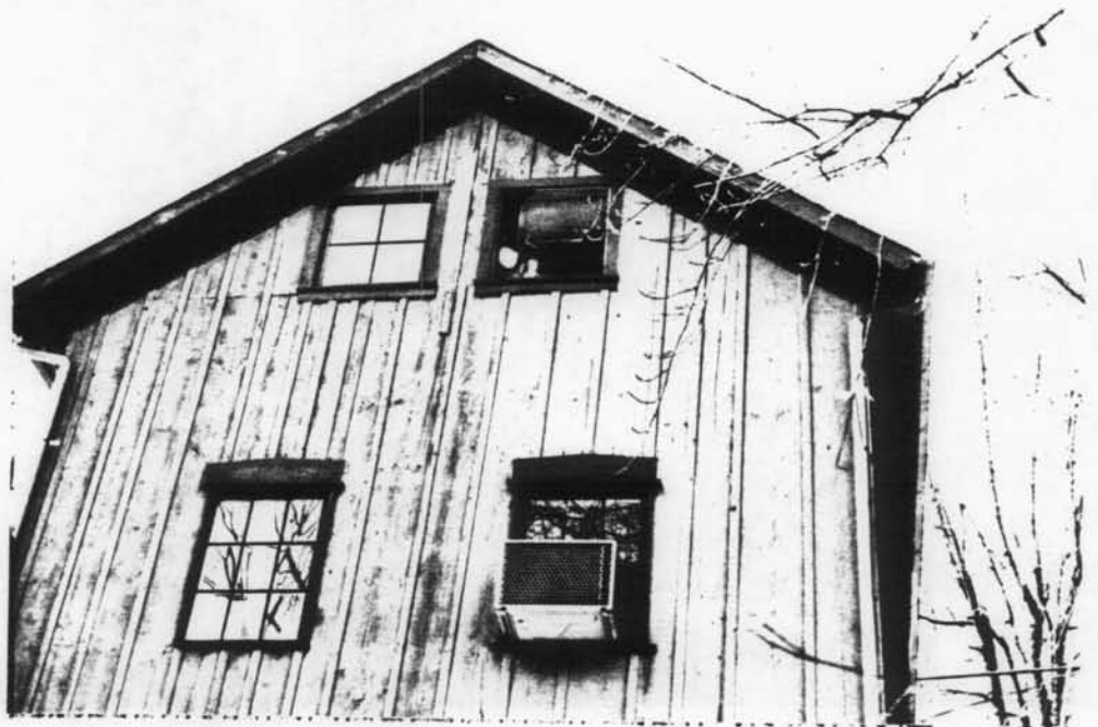
Fig. C-6 Rear elevation after rehab. Windows on first floor retained; board and batten retained. Window in attic converted from single 4-light opening to a split paired unit. Heat pump window units placed in 2 right windows to avoid cuts thru wall.
